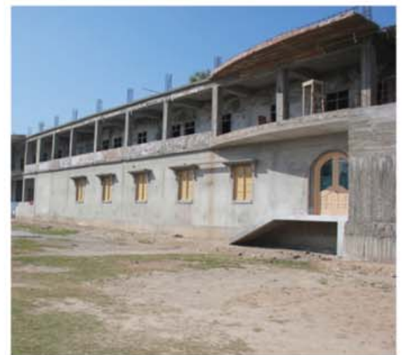
The construction of LaSalle College Faisalabad allows girls – who otherwise had to stop going to school because of Pakistani Legislation - to continue getting junior secondary education.
